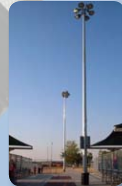
Sports Field Lighting
